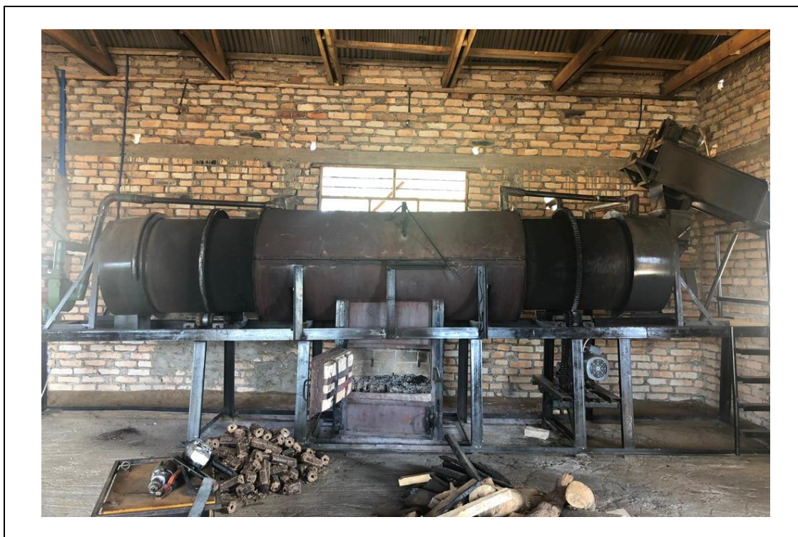
Figure 38 Locally manufactured sawdust carboniser installed at the FWITC
